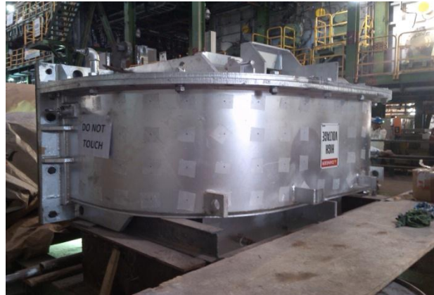
Image 12: High Voltage electrically charged Inductor
